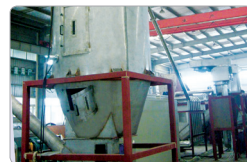
Process weighing system
